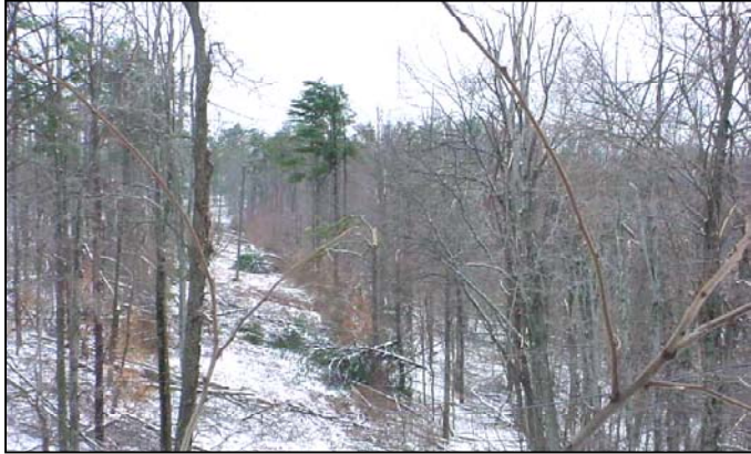
PHOTO 32: Normally Adequate R/W Wasn't Enough to Ward Off Devastation Inflicted by this Ice Storm
