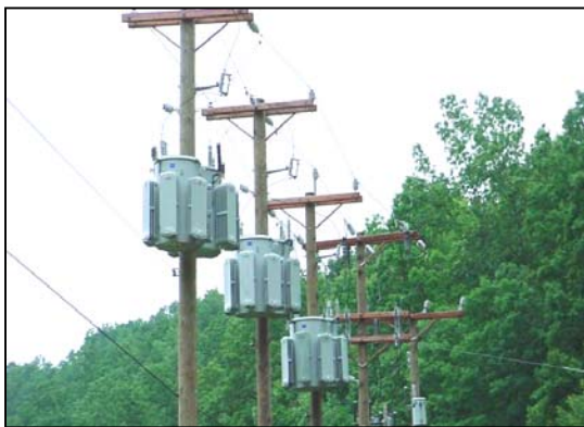
PHOTO 35: 34.5 x 12.4 kV Transformers
