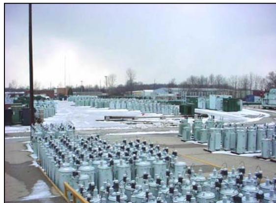
PHOTO 10: KU / LGE Transformer Storage Facility
